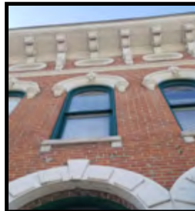
2.a.iv. Roof features and detailing are key characteristics of the Downtown District.
