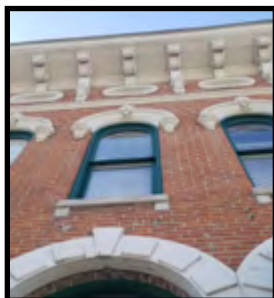
2.a.iv. Roof features and detailing are key characteristics of the Downtown District.
